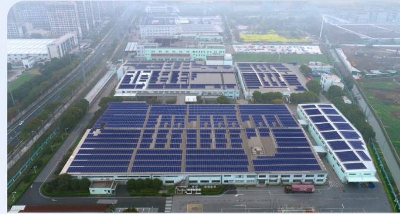
4.58 MW Suzhou CSCEC Proterial C&I Rooftop PV Project
